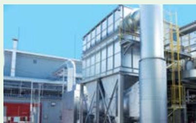
排ガス処理設備 Exhaust-gas treatment facility
